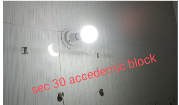
Motion sensor based lights in washrooms of the campus
